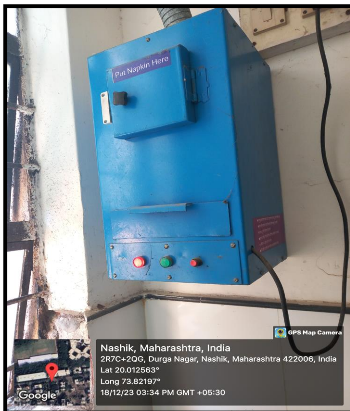
Disposal of biomedical waste
