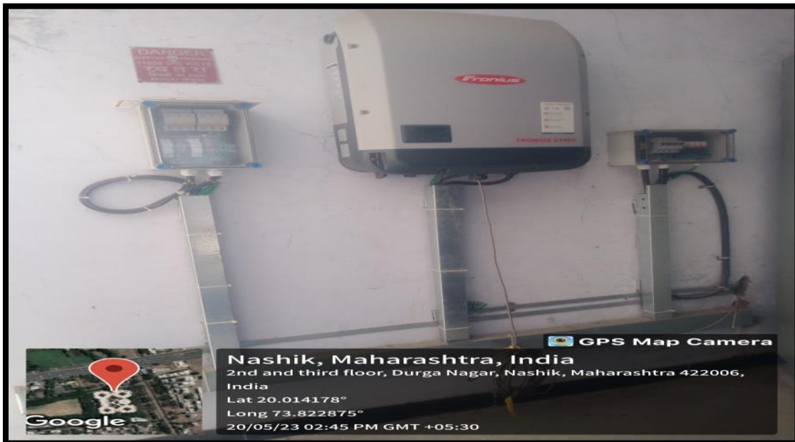
Solar Power Inverter Room
